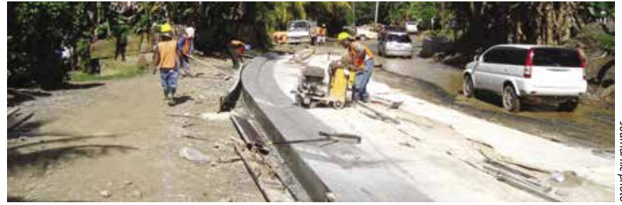
Pacific International staff worked on the Chuuk road and sewer lines project in 2011.
